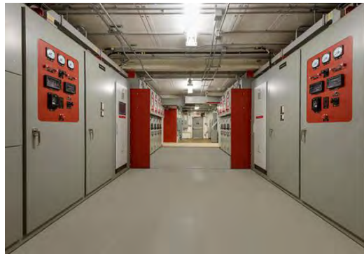
Figure 5-61 Substation switchgear installed
