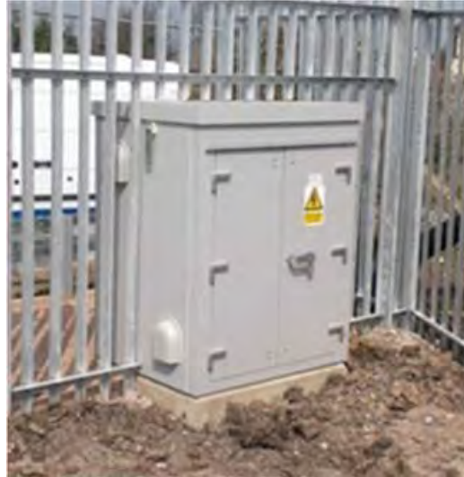
Figure 5-67 Double sided DNO/distribution cubicle
