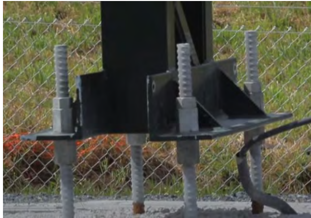
Figure 5-83 Foundation anchor for masts
