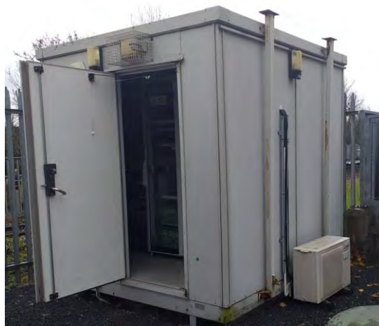
Figure 5-74 Existing TER at Coolmine
